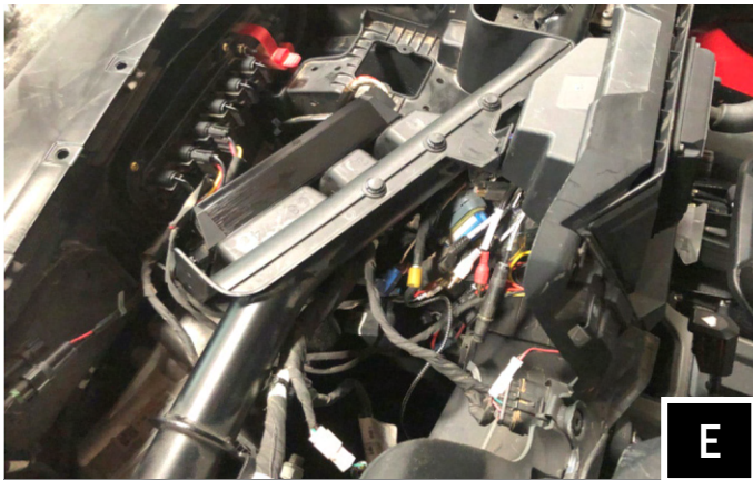
E. Route the MR3 Power Harness and Low Level Harness into the dash. Route the ring terminal end of the MR3 harness to the bus bar.
