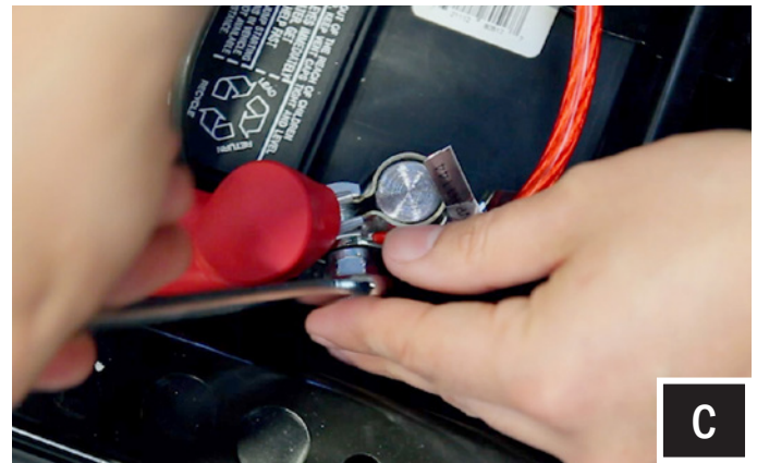
C. Unscrew the factory nut on the positive battery terminal. Install the 2 power cables to the screw on the positive battery terminal. Re-install the factory nut.
