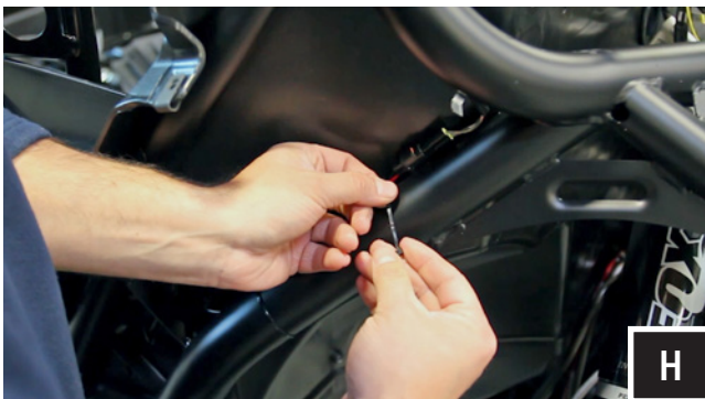
H. Connect the B-H1149 cable to the speaker pods and zip tie all cables to the frame
